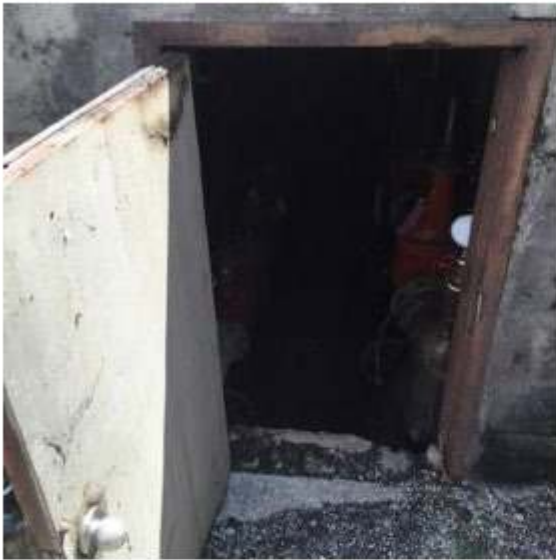
Image 7 - Main Water shut off
