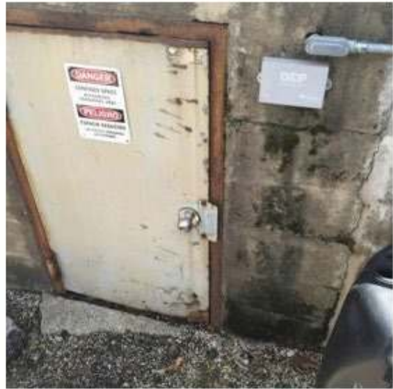
Image 8 – Main water shut off
